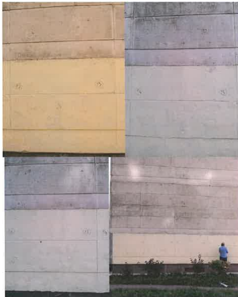
Figure 6. Samples were taken from the North-west orientation façade of building: No12; No13; No14; No15; No16; No17
