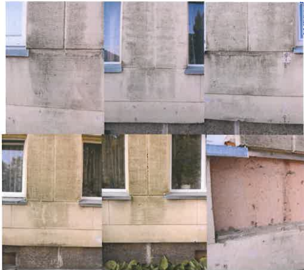
Figure 4. Samples were taken from the North-east orientation façade of building: No1; No2; No3; No4; No5
