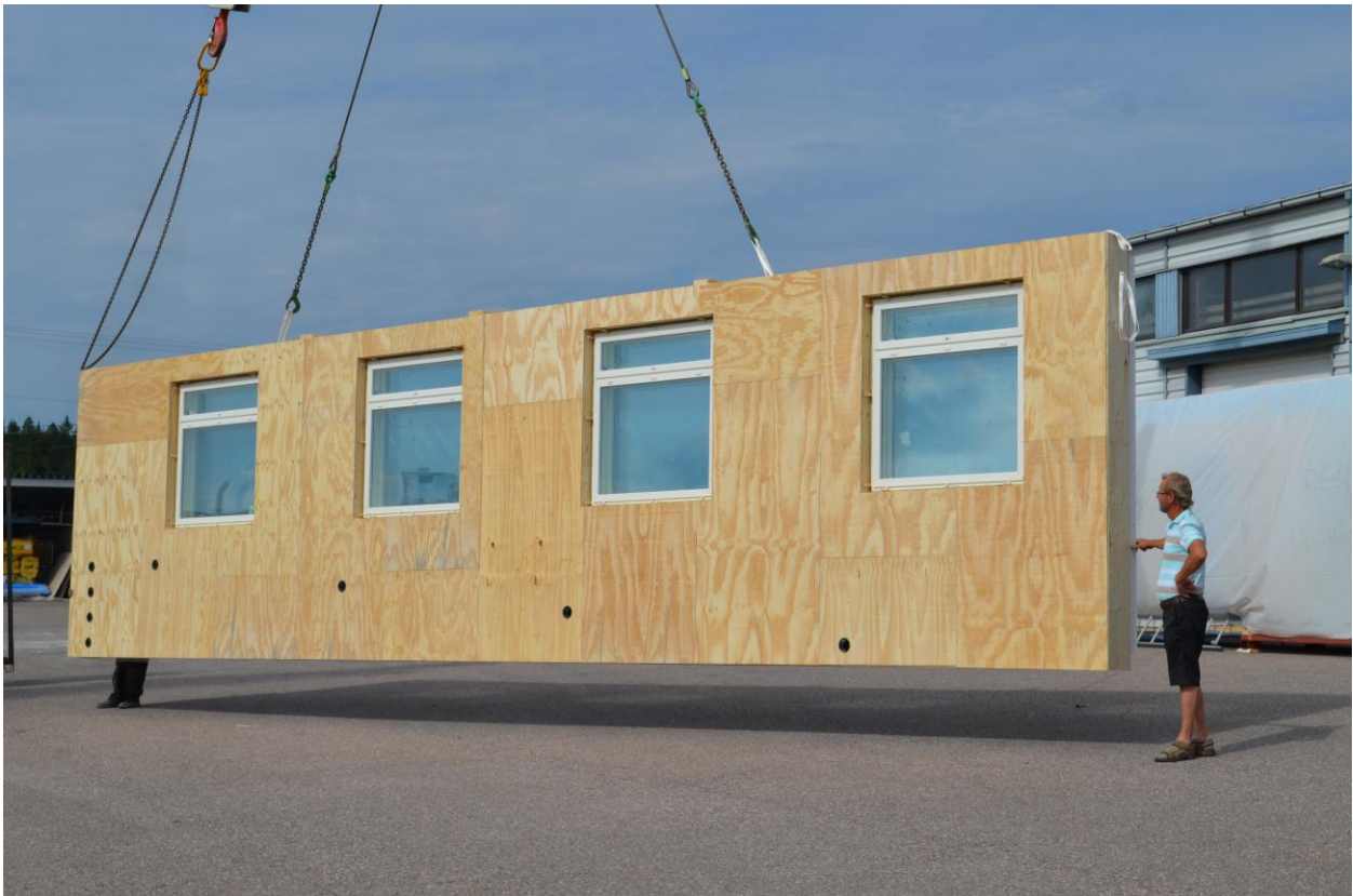
Fig. 3 The elements are transported in horizontal position and will be turned by the crane. The model element was tested at the element factory before the manufacturing was started. The round holes are the ventilation ductwork connections. Photo: Kimmo Lylykangas.
